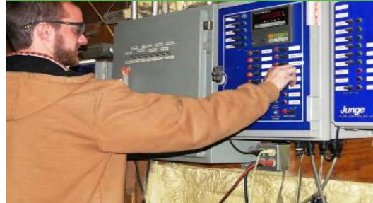
Automated Liquid Blending Controls
